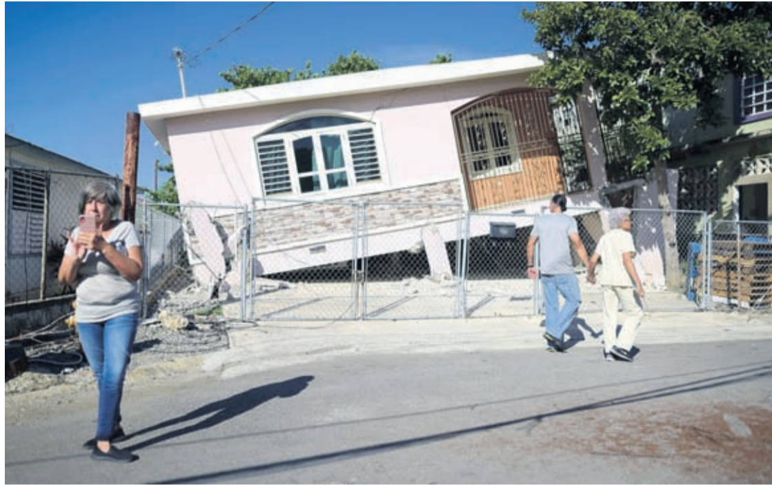
Residents survey damage where a home partially collapsed after an earthquake hit Guánica, Puerto Rico, Monday, Jan. 6, 2020.
